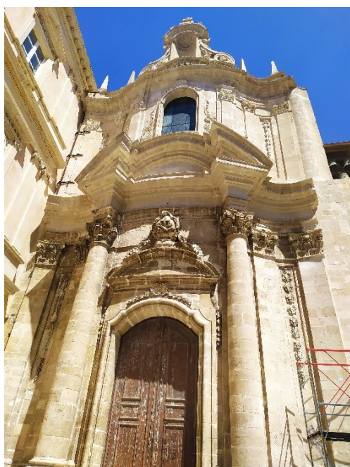
Figure 1 – The façade of the S. Francesco all'Immacolata Church, in the historical centre of Ortigia (SR).
